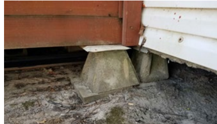
Figure 4. Ineligible dry-stack foundation.
