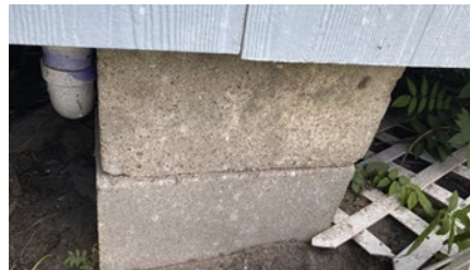
Figure 2. Ineligible dry-stack foundation.
