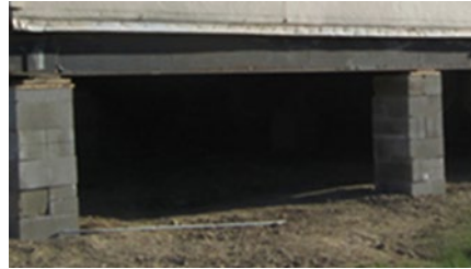
Figure 1. Ineligible dry-stack foundation. No mortar is seen between the blocks.
